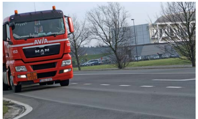
Heavily rutted asphalt pavement, due to heavy traffic and accelerated by high ambient temperatures © FEBELCEM
