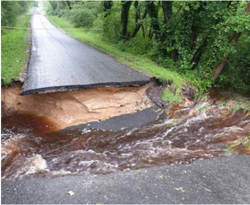
Road damaged after flooding, Gironde (France) © Facebook page of Noaillan
