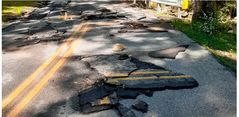
Road damaged after floodwaters, Reading Drive, PA (USA) © Rich Hawk / sauconsorce.com
