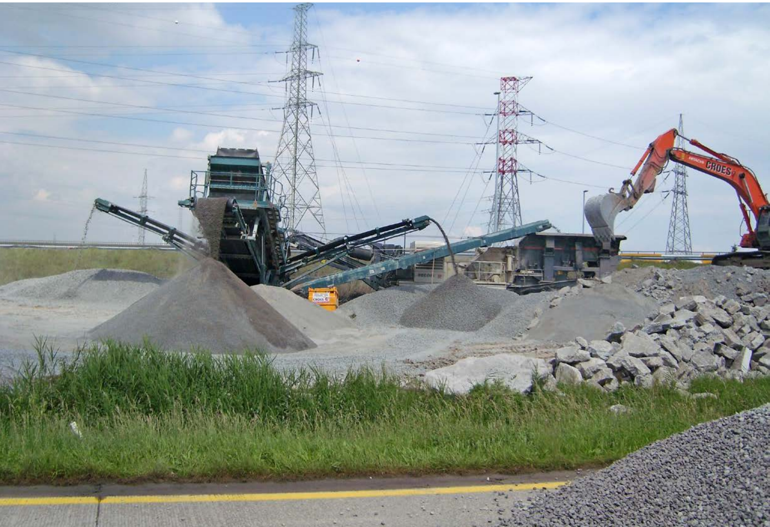
Crushing and sieving installation at motorway N49, Zwijndrecht, Belgium, 2007 © AWW, Flemish Agency for Roads and Traffic
