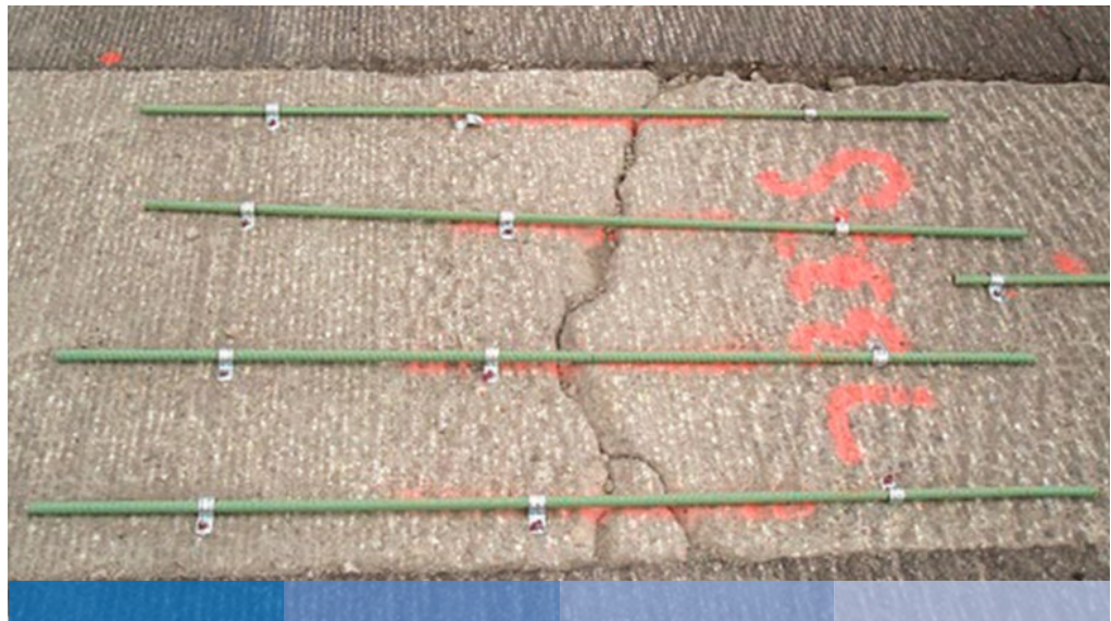
Figure 32. Deformed bars stapled over asphalt crack to prevent reflective cracking. Photo: James Cable, Iowa State University.
