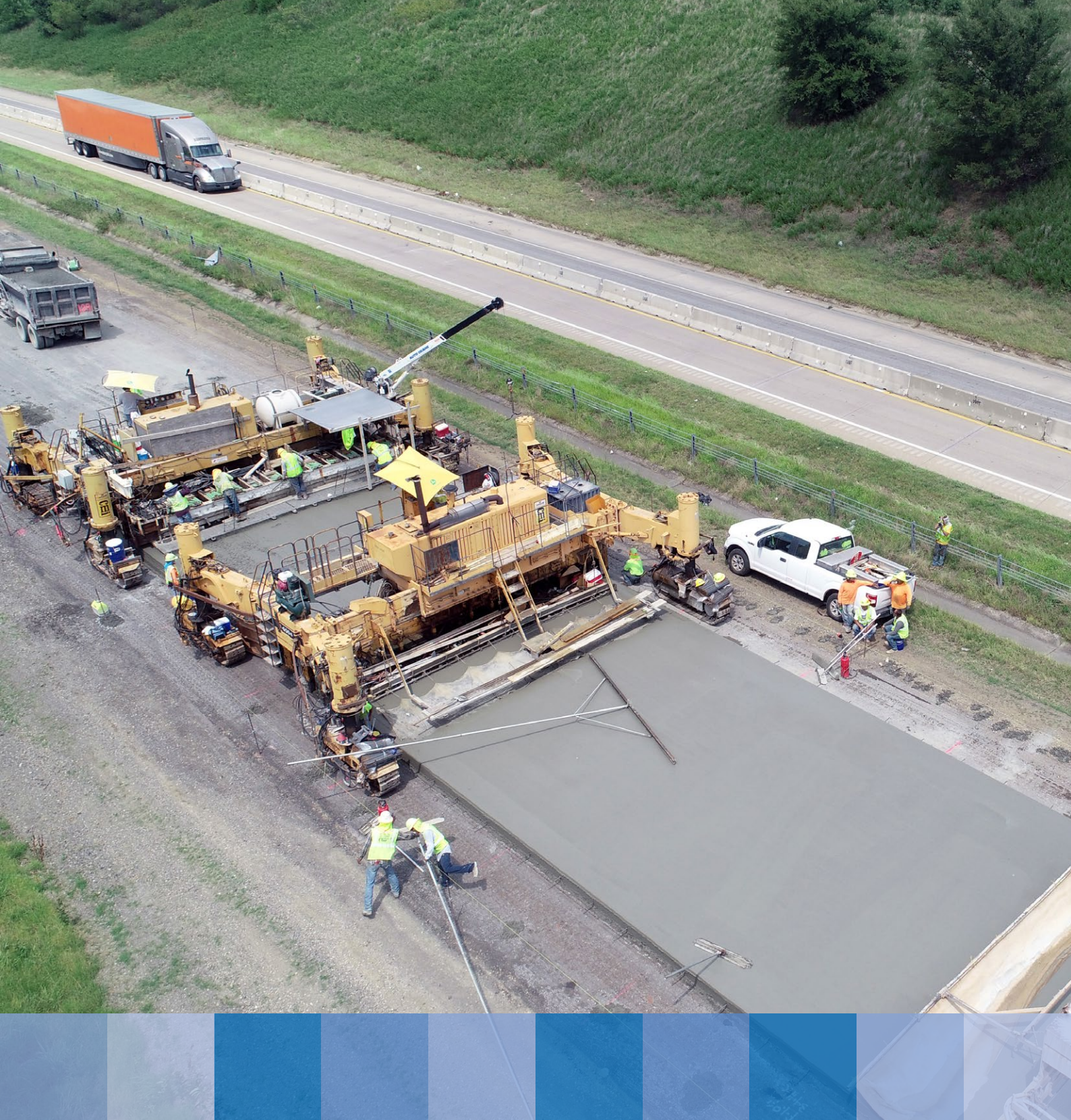
Unbonded concrete overlay of asphalt pavement on U.S. Route 69 near Caddo, Oklahoma, U.S., 30 cm thick. Photo: ACPA.
