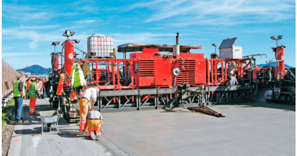
Figure 11. Example of the NOBI - the "New Austrian Concrete Overlay Method" bonded concrete inlay of concrete on the A1 (Spalt 2015).
