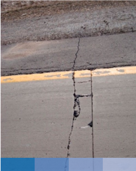
Figure 7. Example of asphalt pavement transverse crack reflecting through thin concrete overlay. Photo: J. Vandebossche, University of Pittsburgh.
