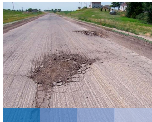
Figure 9. Thin asphalt and base material exposed after milling (Fick, et al. 2021).
