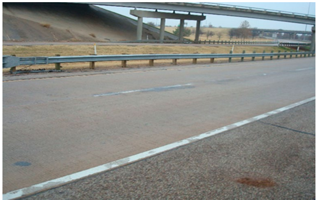
Figure 12. Bonded CRC over CRCP (US 281 in Texas, USA) - 2018 photo of 2002 construction. Photo: Mark Snyder, PERC, LLC.
