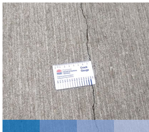
Figure 28. Reflective cracking in COA-B without fibers (left) and with macrofibers (right). Photos: Snyder and Associates.
