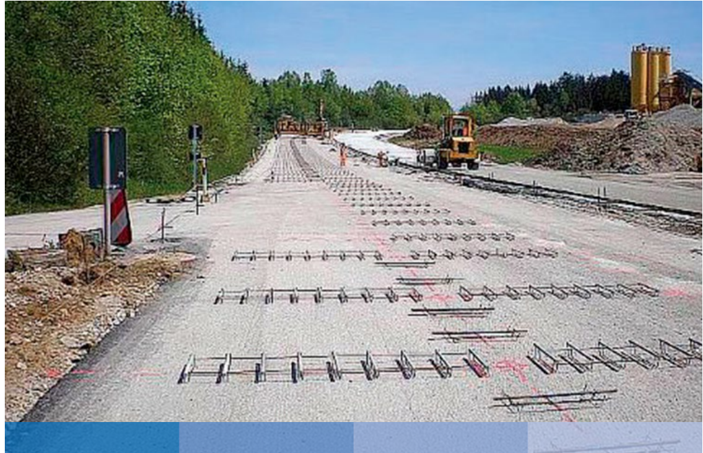
Figure 38. Construction of doweled and tied COA on Agg near Munich, Germany (Riffel, 2010).
