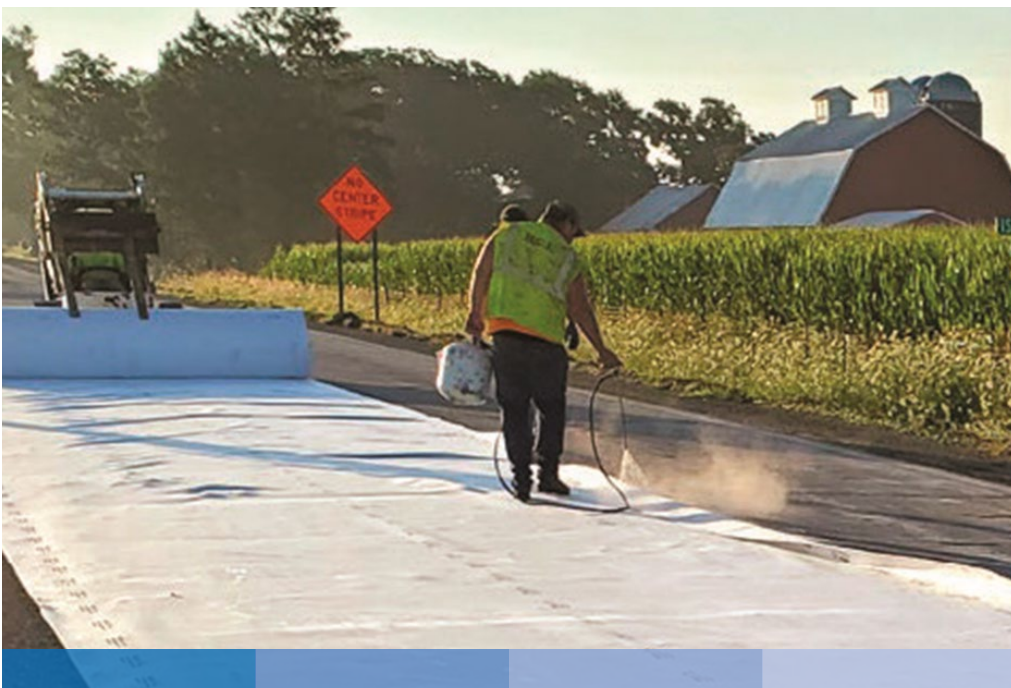
Figure 25. Use of adhesive to anchor geotextile fabric. Photo: Dan King, Iowa Concrete Paving Association.
