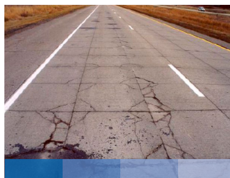
Figure 31. 7.5 cm bonded concrete overlay of 25 cm asphalt, 1.8m panels (left) and 1.2m panels (right), 6 years of service, ~6M 80-kN axle loads. Photos: Julie Vandebossche, Univ. of Pittsburgh)
