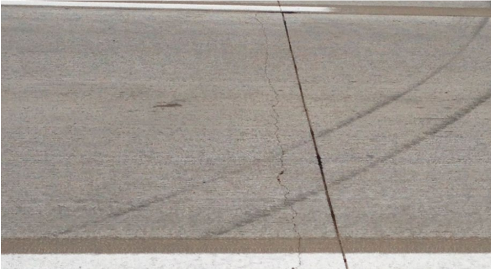
Figure 13: Reflection of underlying pavement joint through bonded concrete overlay. Photo: Todd LaTorella, MO-KS Chapter of ACPA.
