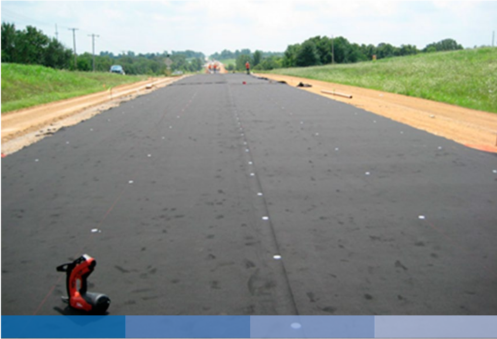
Figure 24. Overlapping sections of nonwoven geotextile fabric, anchored with nails and washers. Photo: ACPA.
