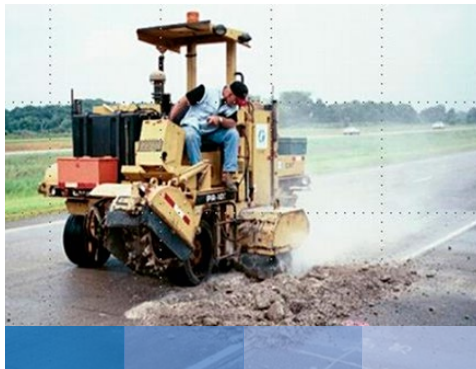
Figure 44. Techniques for removing thin concrete overlay panels. Photos: Julie Vandembossche, Univ. of Pittsburgh.
