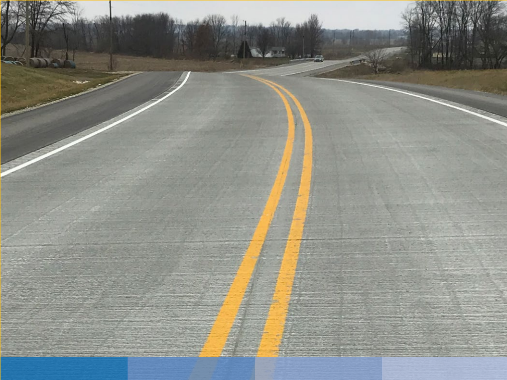
Concrete overlay of asphalt-surfaced road in Daviess County, Indiana, U.S., 2019, 15 cm thick. Photo: ACPA.
