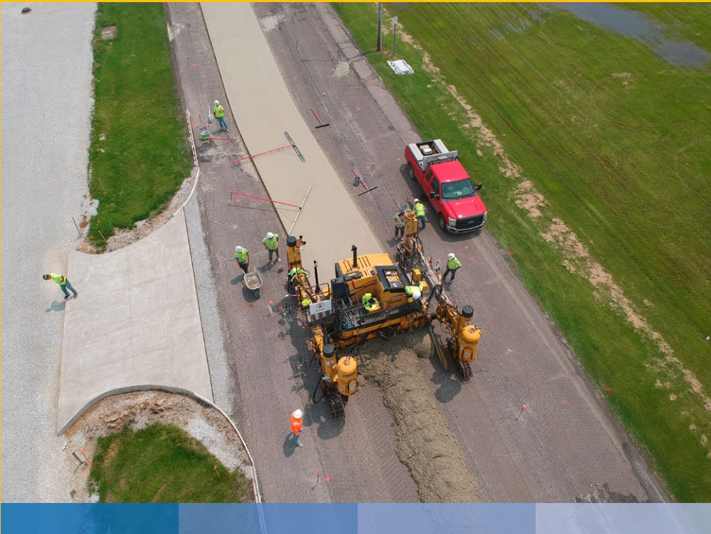
Fiber-reinforced concrete overlay of asphalt-surfaced local road Grant County, Indiana, U.S., 2020, 15 cm thick. Photo: ACPA.
