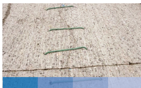
Figure 15: Use of reinforcing steel over tight longitudinal cracks in existing concrete before placing bonded concrete overlay. Photo: Brent Burwell, OK-AR Chapter of ACPA.
